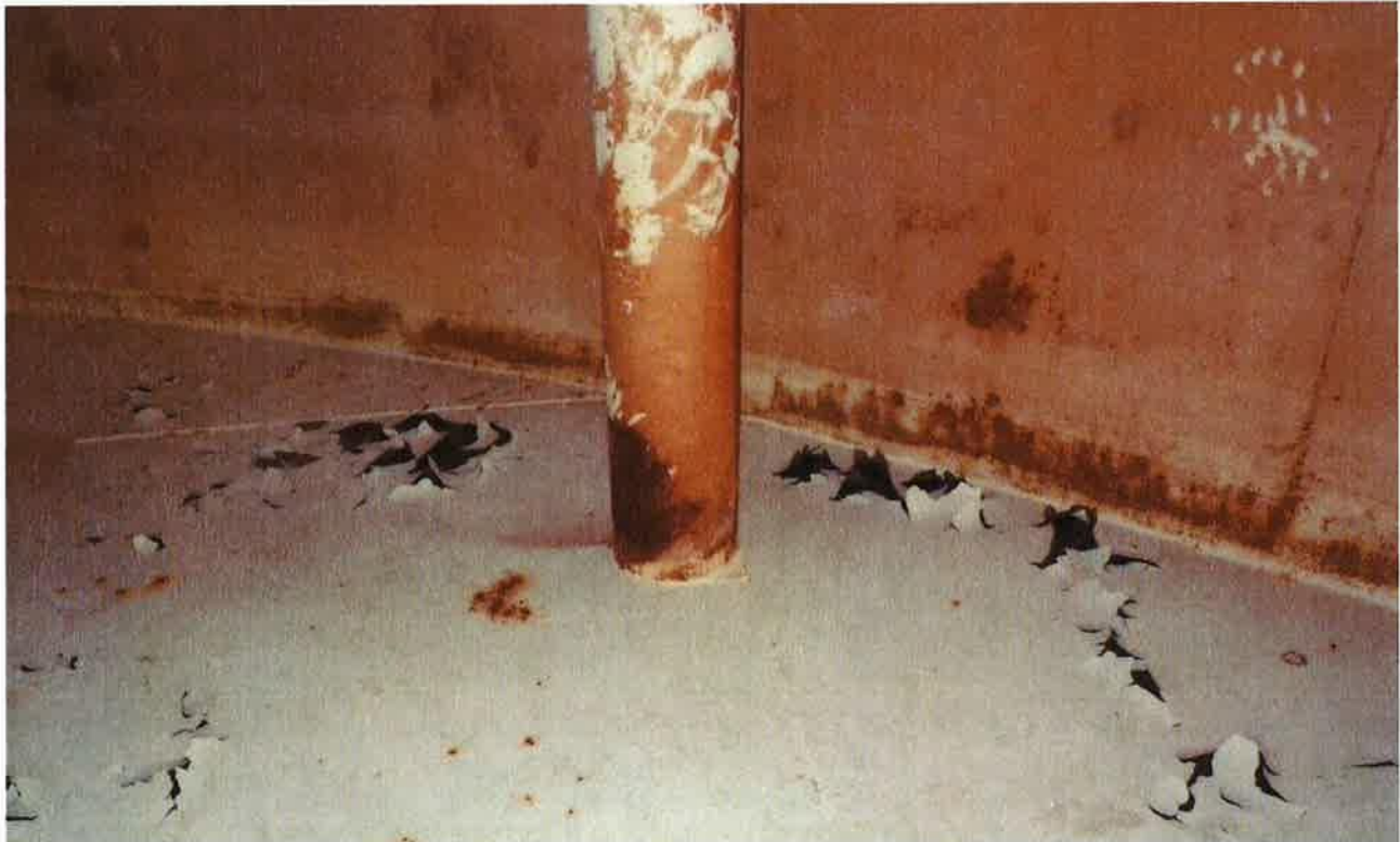
74. Peeled coating on floor near inlet pipe.
