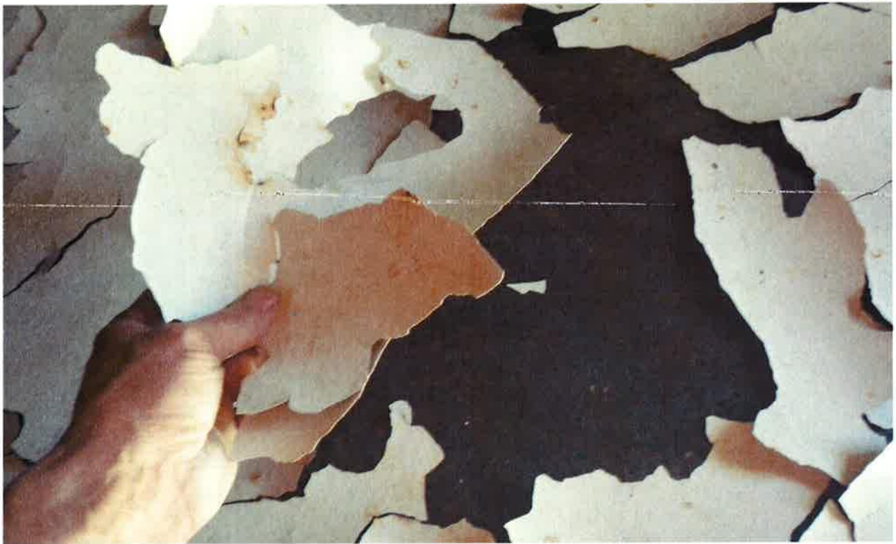
73. Peeled coating on floor.
