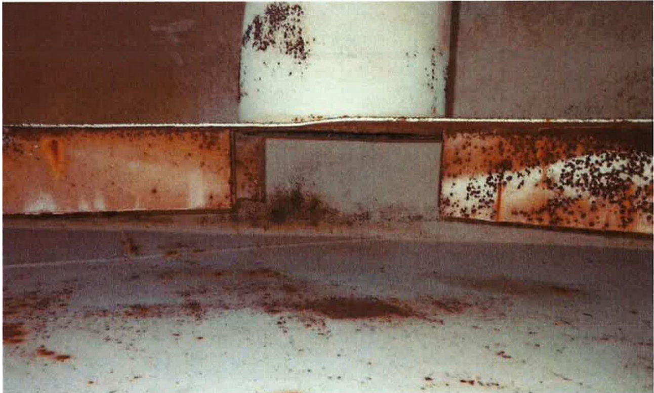
68. Outlet pipe and anti-vortex assembly.
