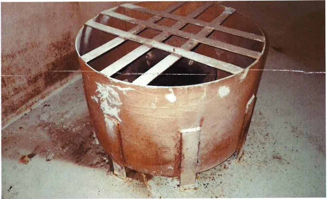
79. Outlet pipe shroud.
