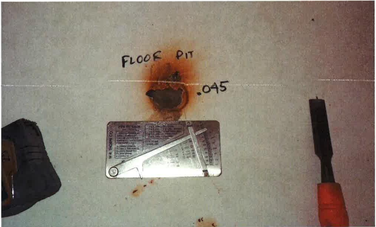
71. Pitting on floor.
