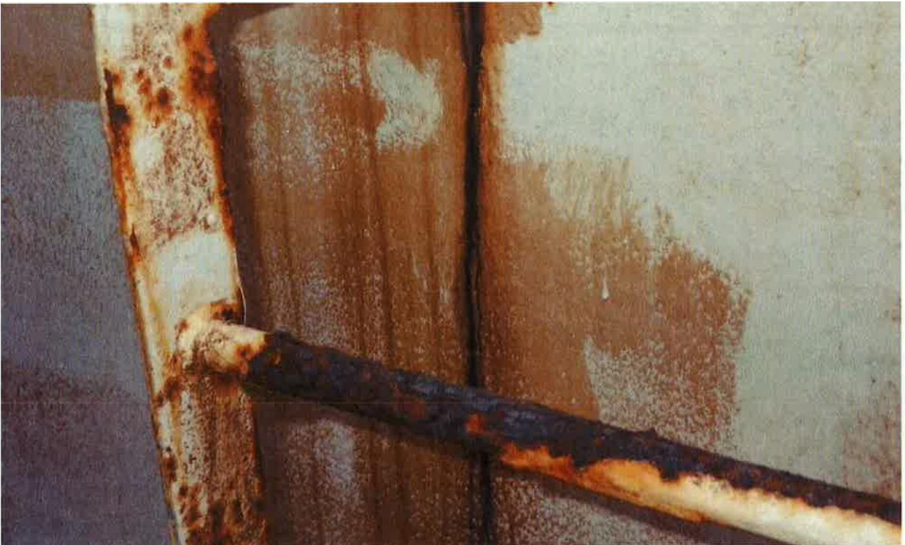
70. Corrosion and metal loss on interior container ladder.
