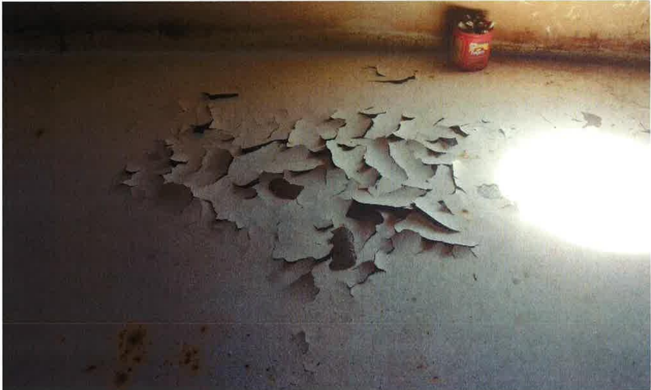
72. Peeled coating on floor.
