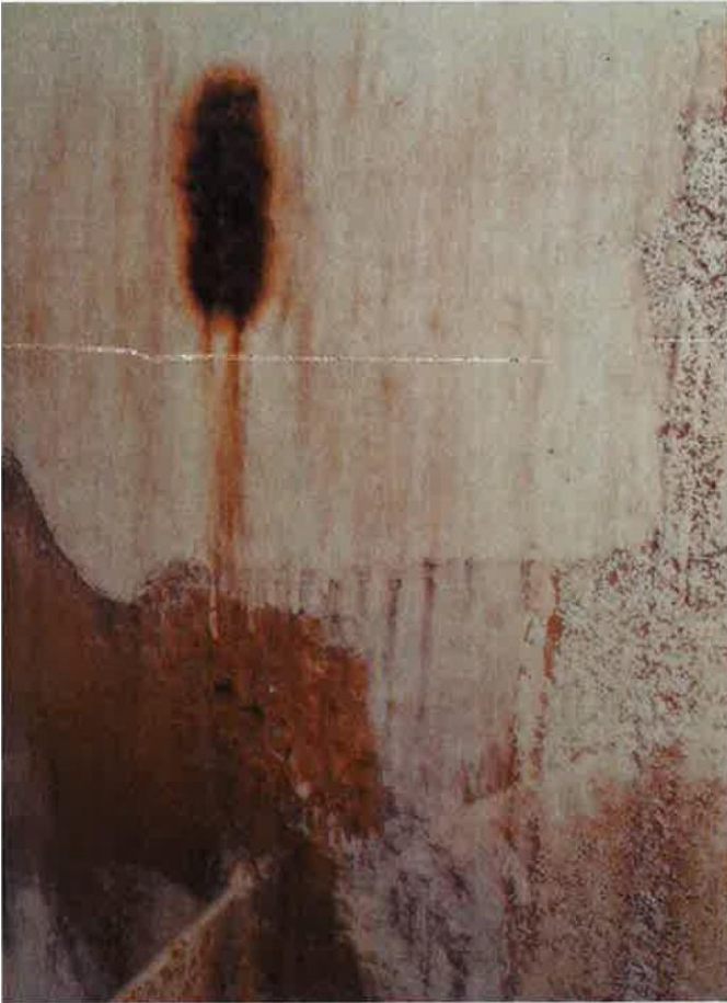
59. Area on shell damaged from exterior welding.
