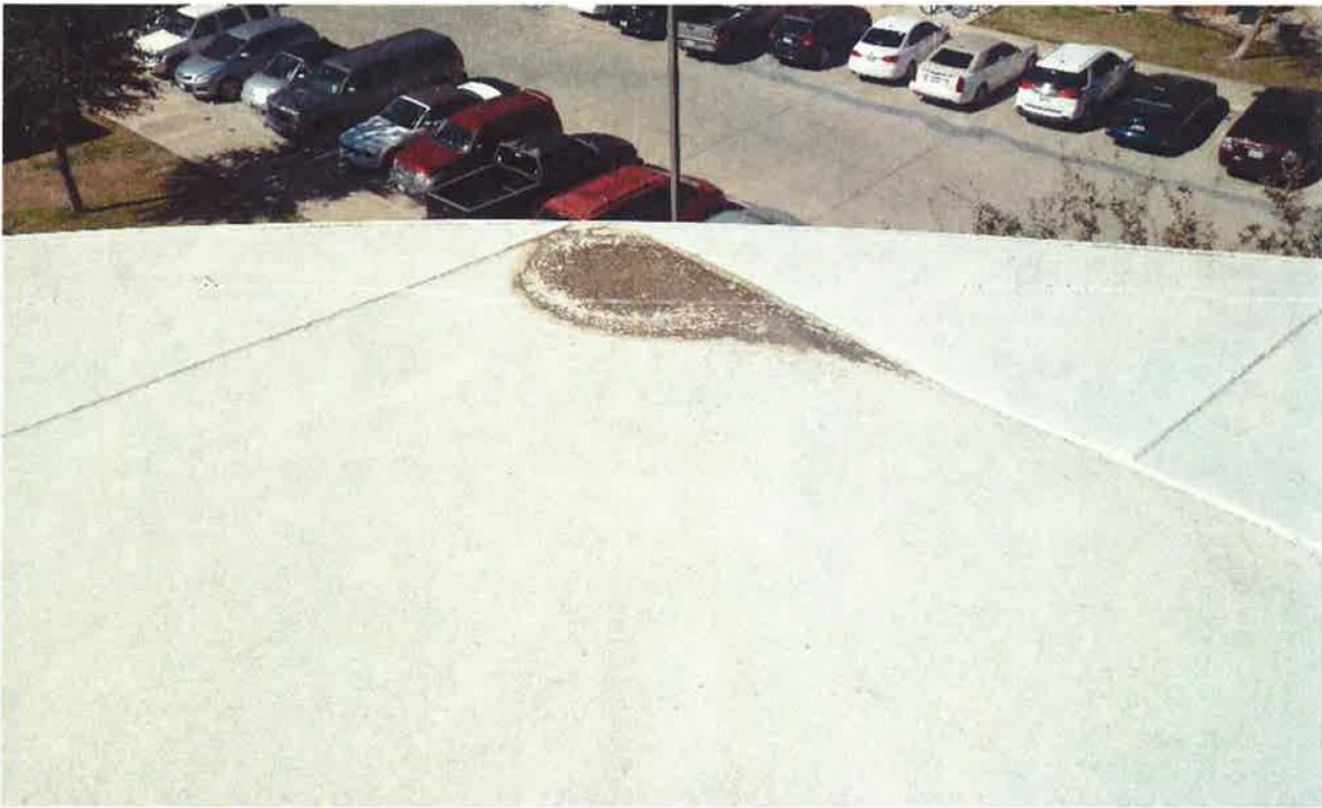
41. Ponding near roof perimeter .
