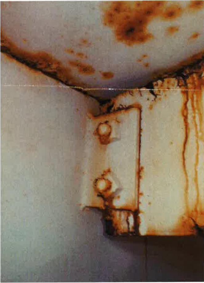
51. Corrosion and metal loss at rafter-to-clip connection.
