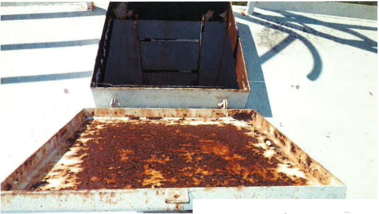
45. Roof manhole. Note corrosion on cover.
