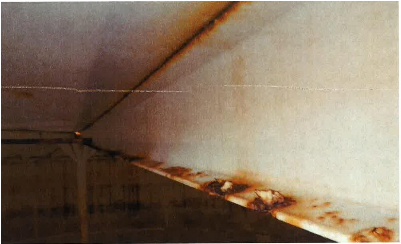
53. Corrosion and metal loss on roof rafter.
