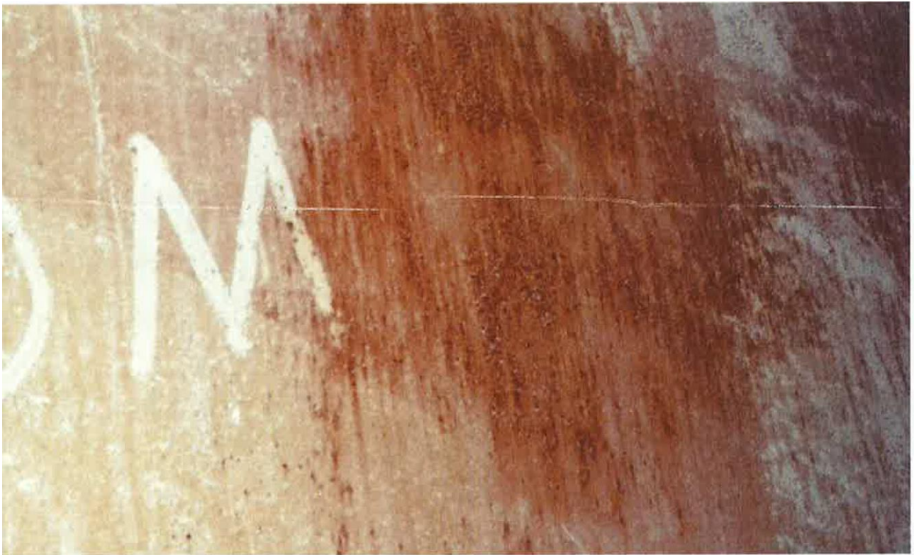
57. Corrosion on shell.
