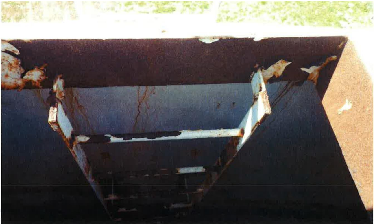
46. Roof manhole and interior ladder. Note corrosion.
