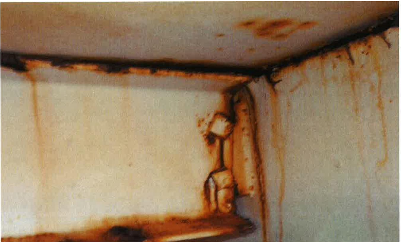
52. Corrosion and metal loss at rafter-to-clip connection.
