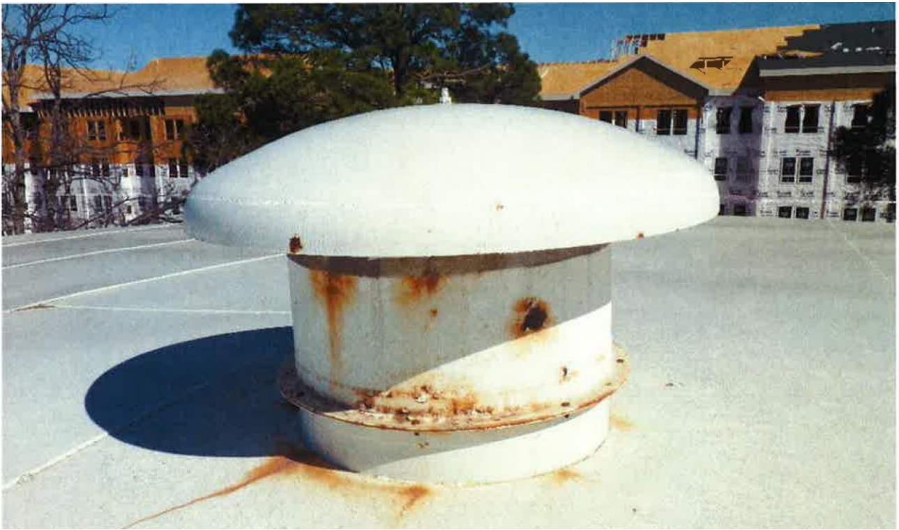
47. Roof vent. Note corrosion.
