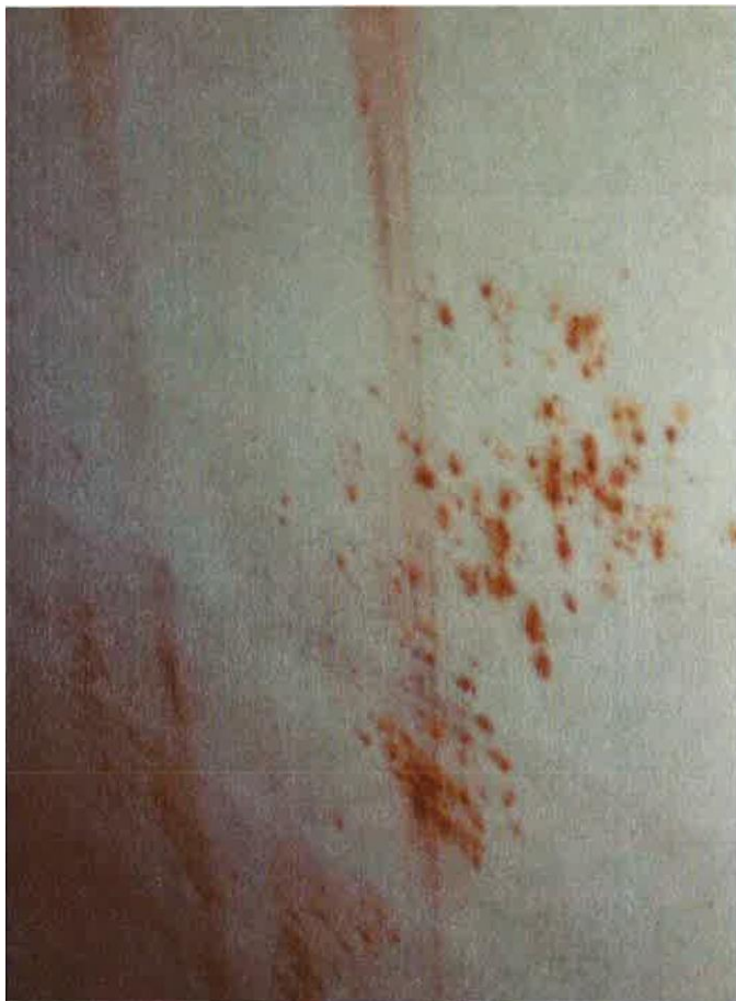
58. Corrosion on shell.
