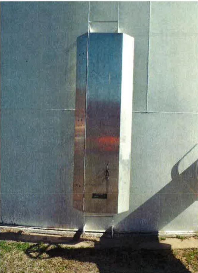
34. Ladder vandal deterrent.
