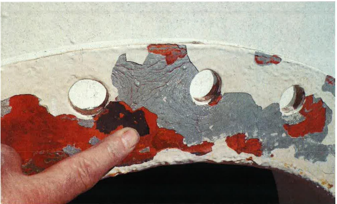
24. Peeled coating and metal loss on shell manhole flange.
