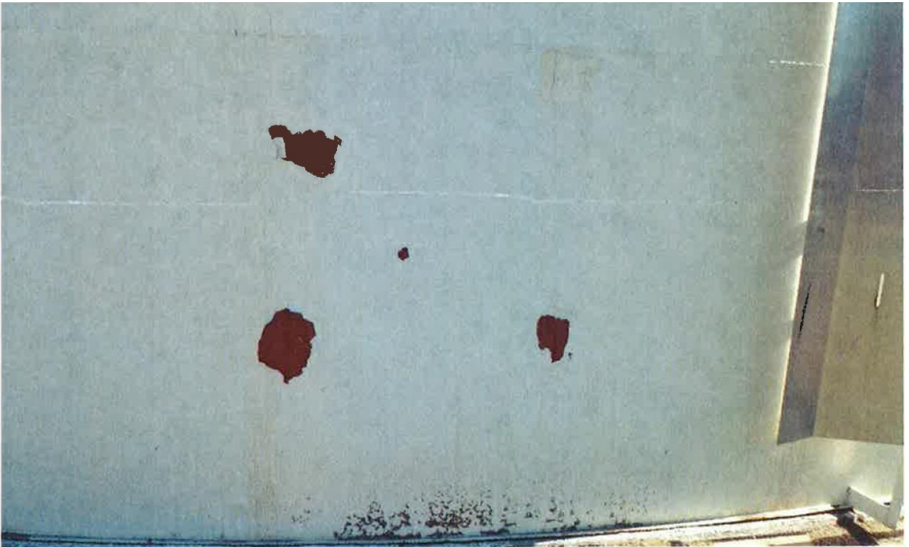
25. Peeled coating on shell.
