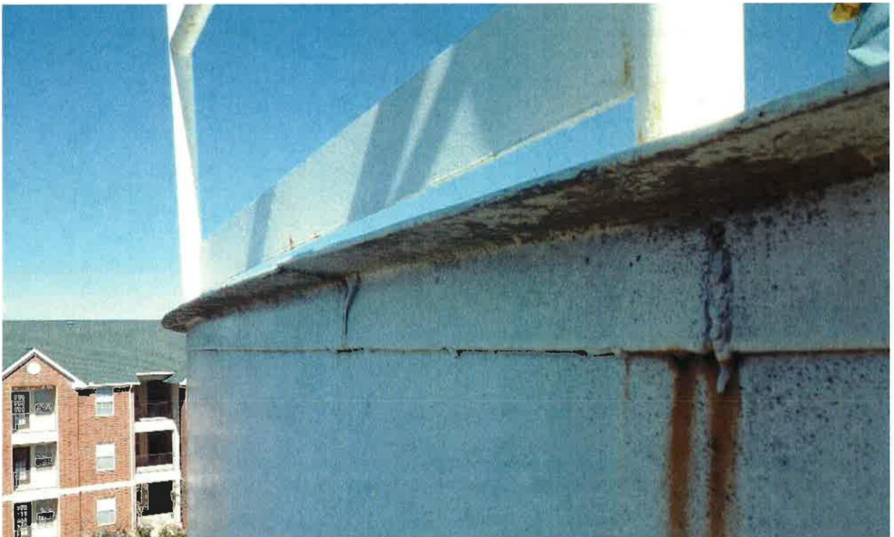
32. Top shell angle and gap between safety railing toe bar and roof.
