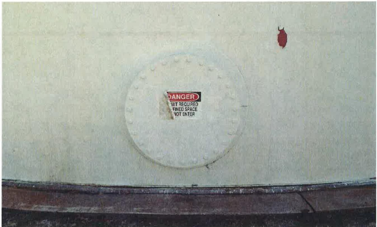
22. Shell manhole. Note "Confined Space" sign on shell manhole cover.
