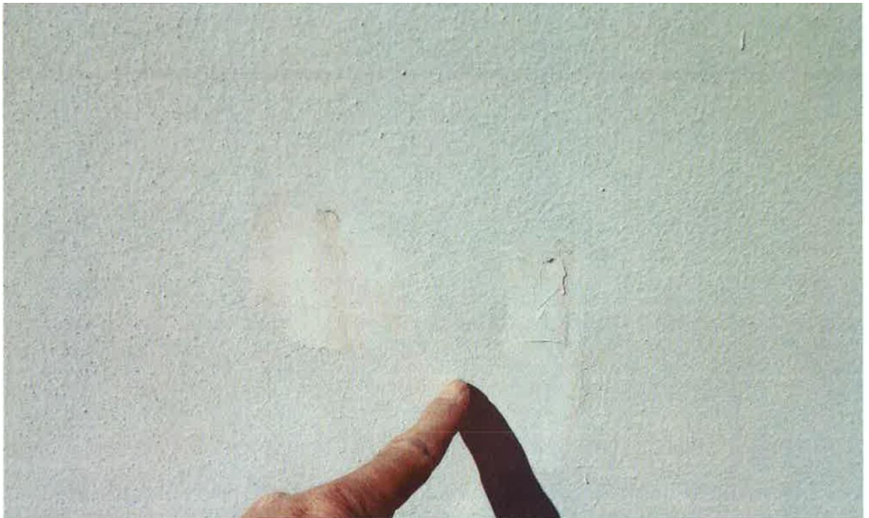
28. Caulked areas on shell.
