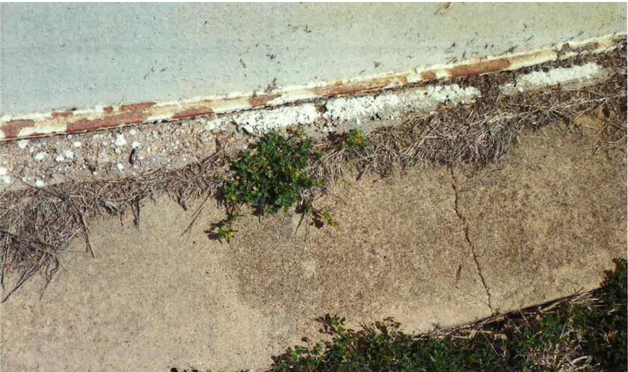
12. Bottom plate and foundation. Note vegetation.
