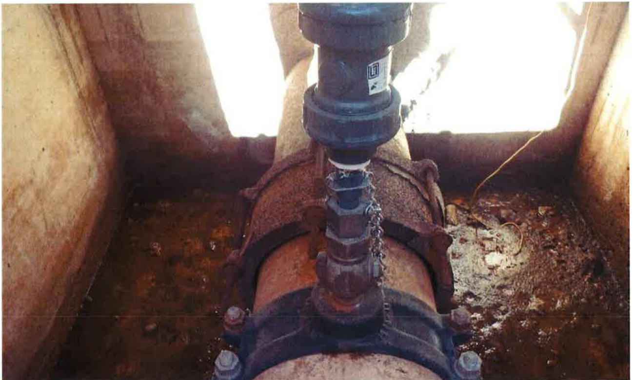
8. Piping in valve vault.
