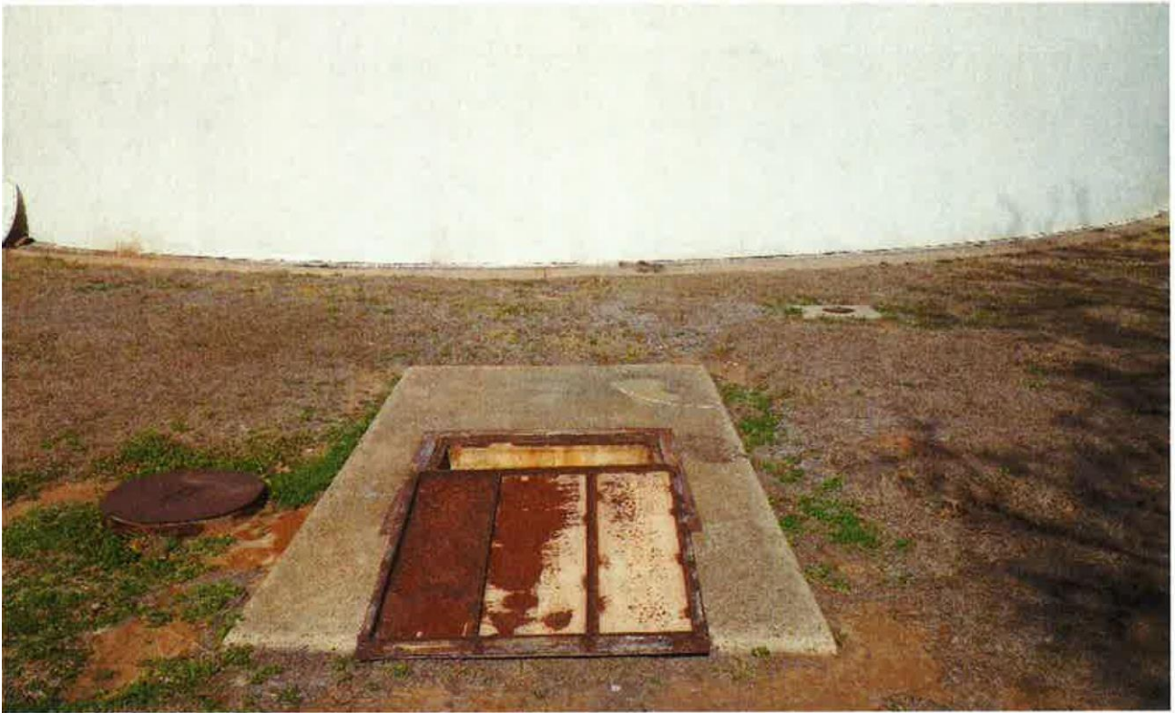
5 . Valve vault exterior.
