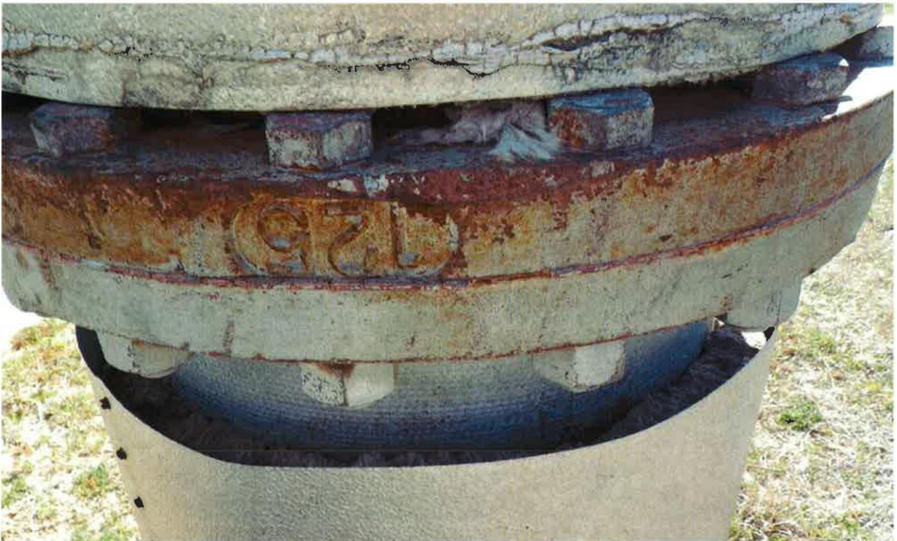
20. Flange on outlet pipe.
