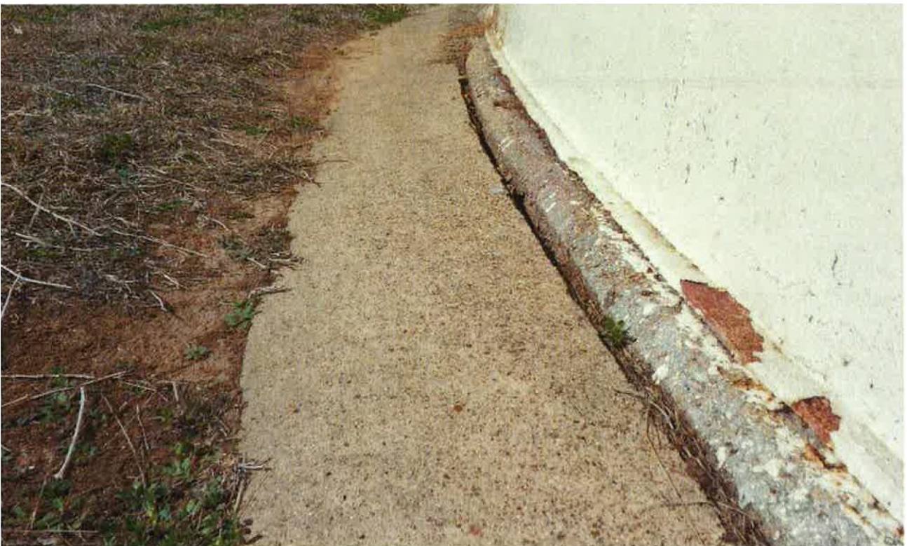
14. Bottom plate and foundation. Note corrosion on bottom plate.
