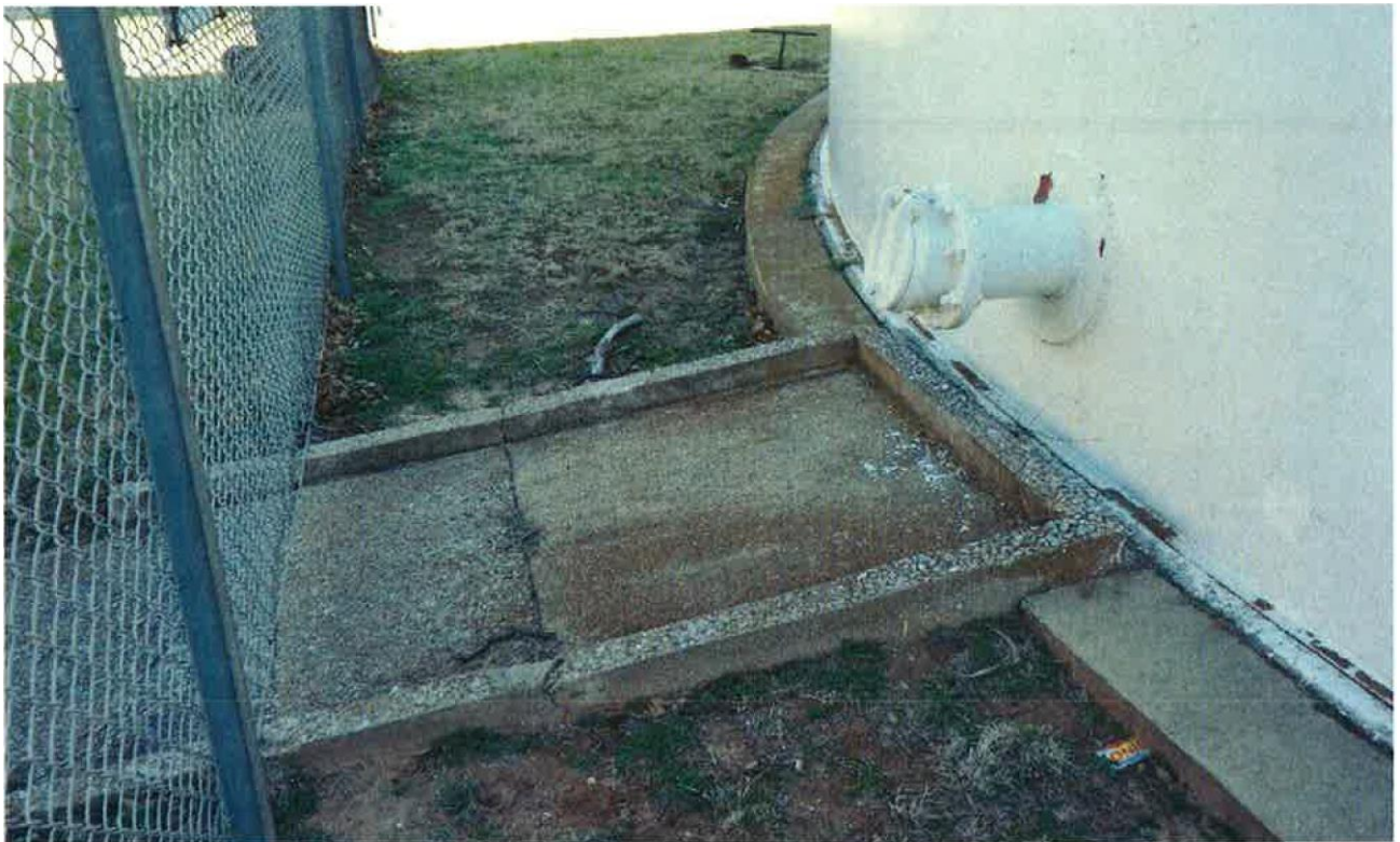
16. Overflow pipe and splash pad.
